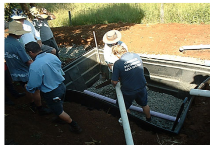
Underdrain and gravel bed
